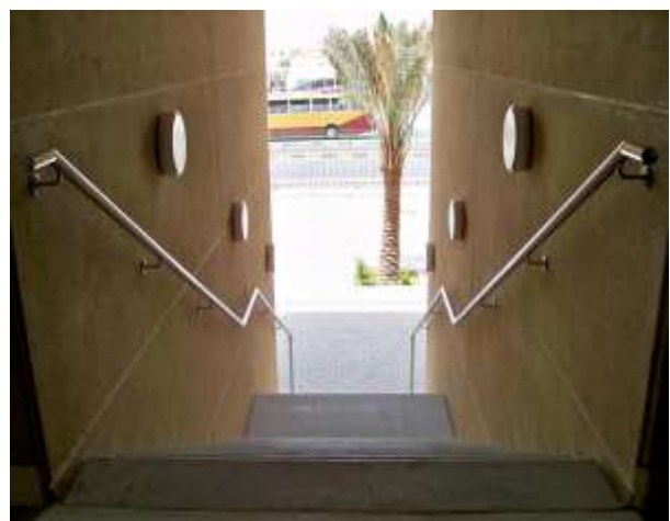
Wall mounted handrails
