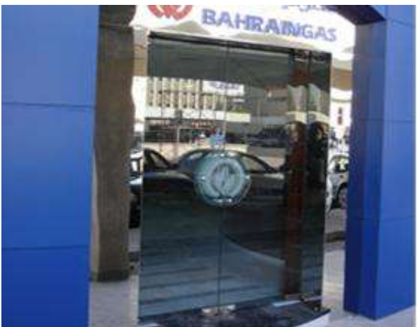
Stainless steel door frame cladding
