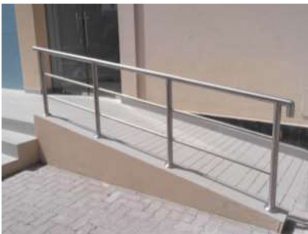
Stainless steel ramp railing
