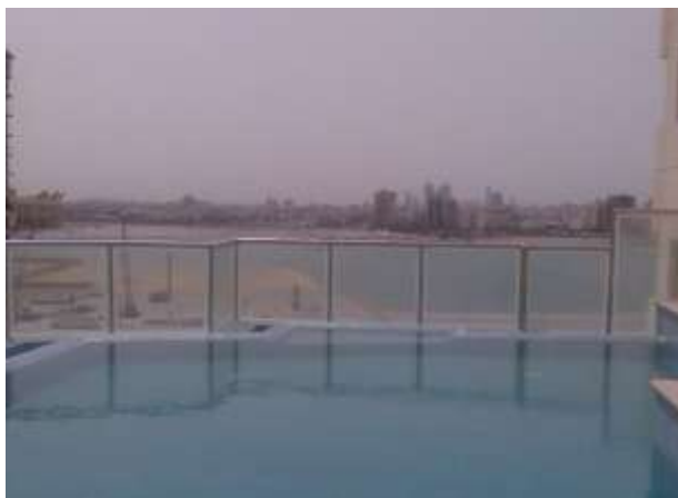
Swimming pool safety railing
