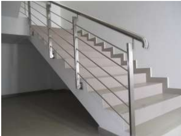
Stainless steel side fixed railing
